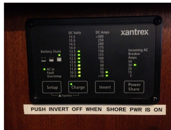
CLOSE UP VIEW OF THE INVERTER PANEL
