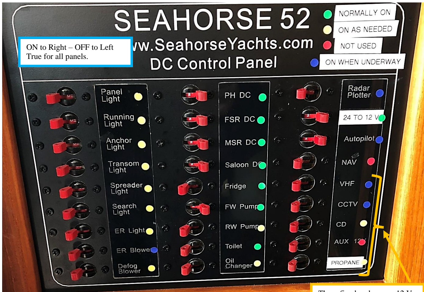
These five breakers are 12 V and need the 24 to 12 V breaker on to get power.
