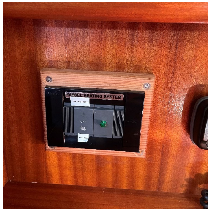
Main on/off switch for furnace. Located above outboard side of nav station.
