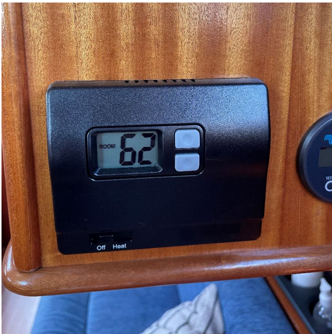
Furnace thermostat (okay to leave set to "heat"). Located above forward end of nav station.
