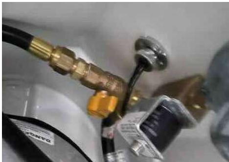
BBQ Isolation Valve (yellow handle). Shown here in off position. Turn inline to run BBQ.
