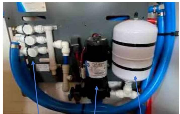
Tank Selection Valves"
