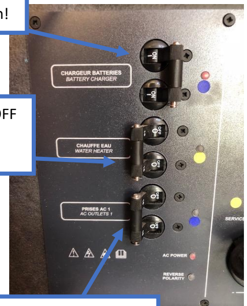
AC Outlets Breaker
