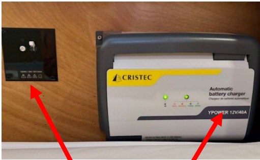
GFI Breaker and Battery Charger
