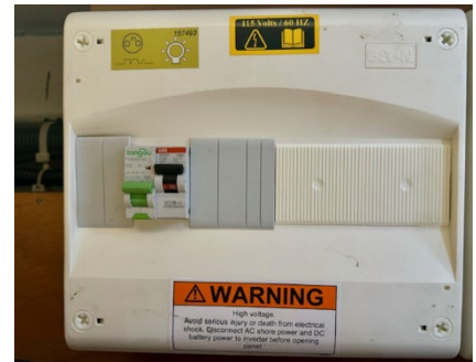
Aft cabinet AC Ground Fault Breaker
