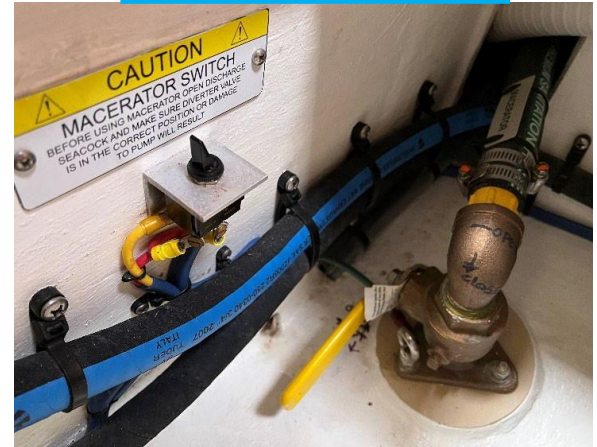
Macerator Through-hull Valve and Pump Switch
