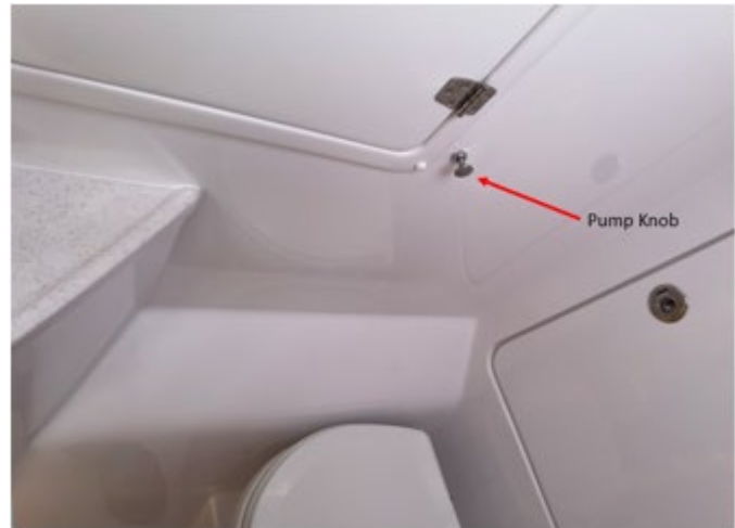
Starboard Shower Pump
