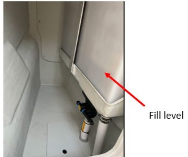
Starboard Blackwater Holding Tank
