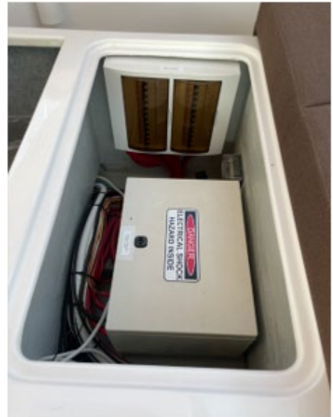
12V DC Breaker Panel
